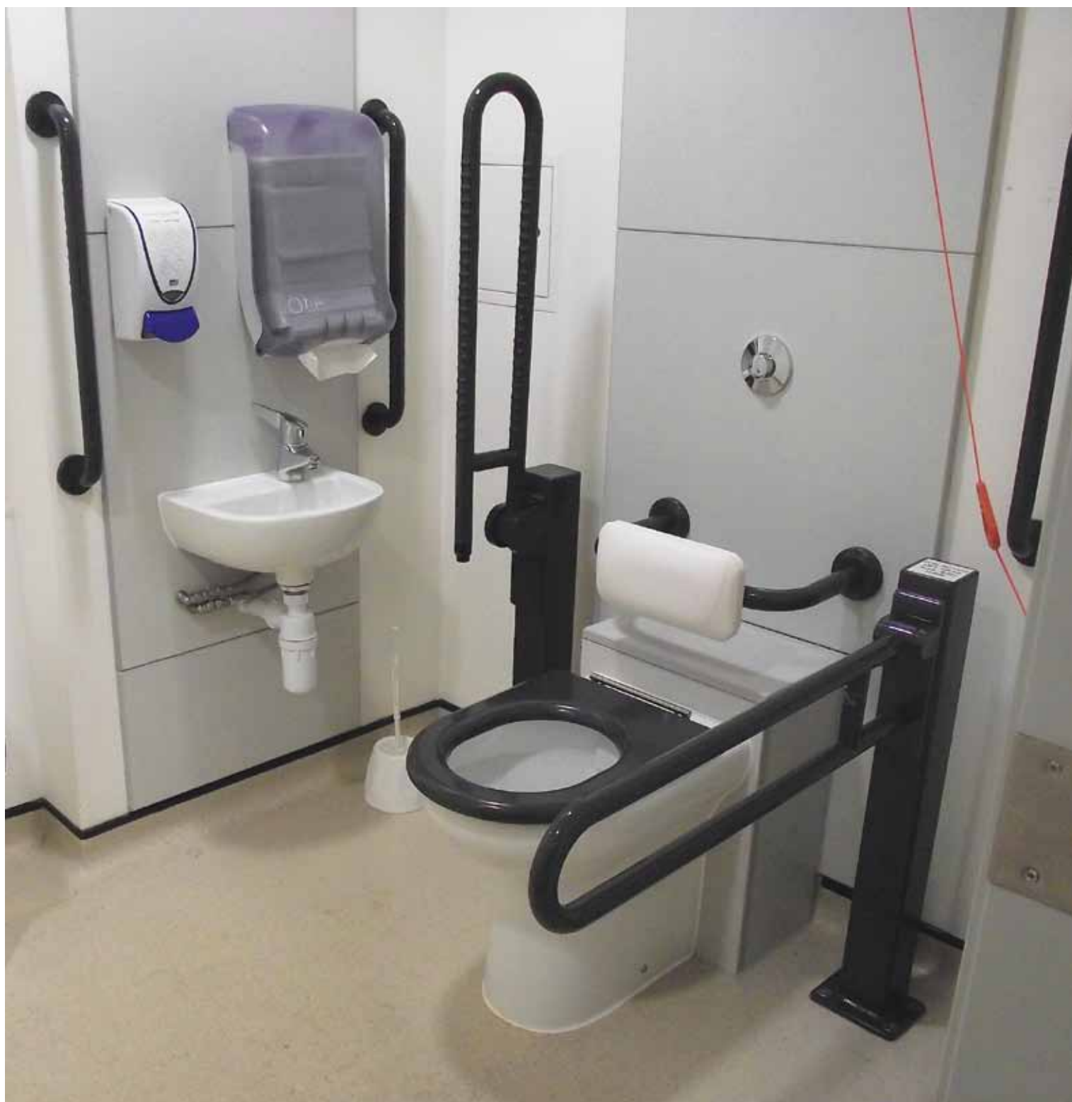
Above: Compact rimless 45cm back to wall WC pan with reinforced ring seat and 38cm basin installed at the Queen Alexandra Hospital Portsmouth
